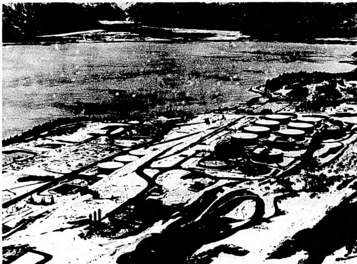
Port Valdez, showing construction progress on the 510,000-barrel storage tanks. Eighteen of these tanks will be built to hold oil from Prudhoe Bay until it can be fed to tankers, at four berths now under construction, for shipment to ports along the west coast of the United States.
