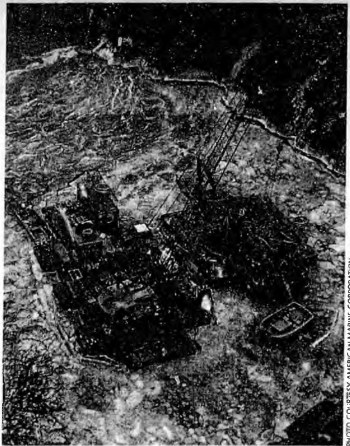
Sitka Blue Lake Hydroelectric Project
