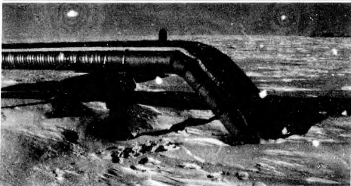
The Milne Point Oil (rear) and Products (front) pipelines connect the Milne Point Development, east of Prudhoe Bay, to the Kuparuk and Oliktok Pipeline Systems, respectively, approximately 10 miles to the south.
