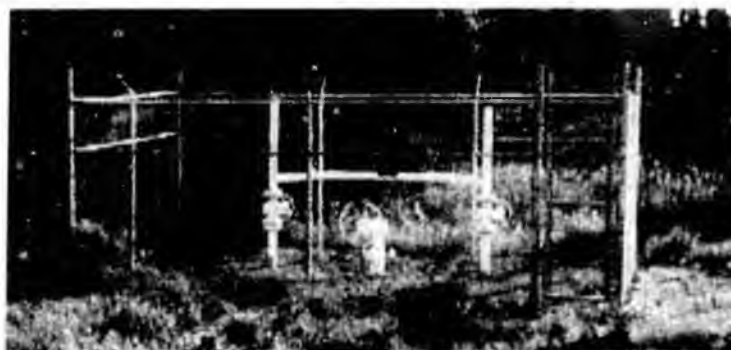
The KKPL valves are enclosed in fencing, locked, and marked with warning signs to inform the public and protect equipment.
