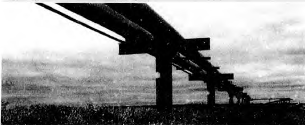
VSMs for the Alpine pipelines are marked with reflector tape for public safety.
