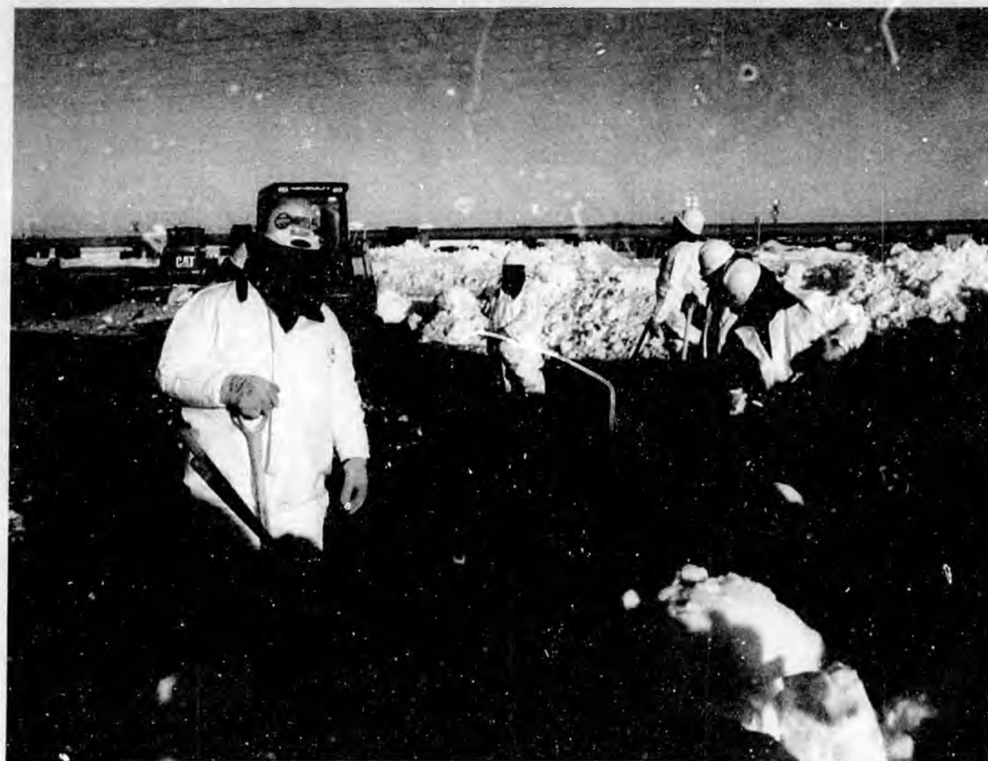
Spill Clean up—Haz Mat Suits on the tundra
