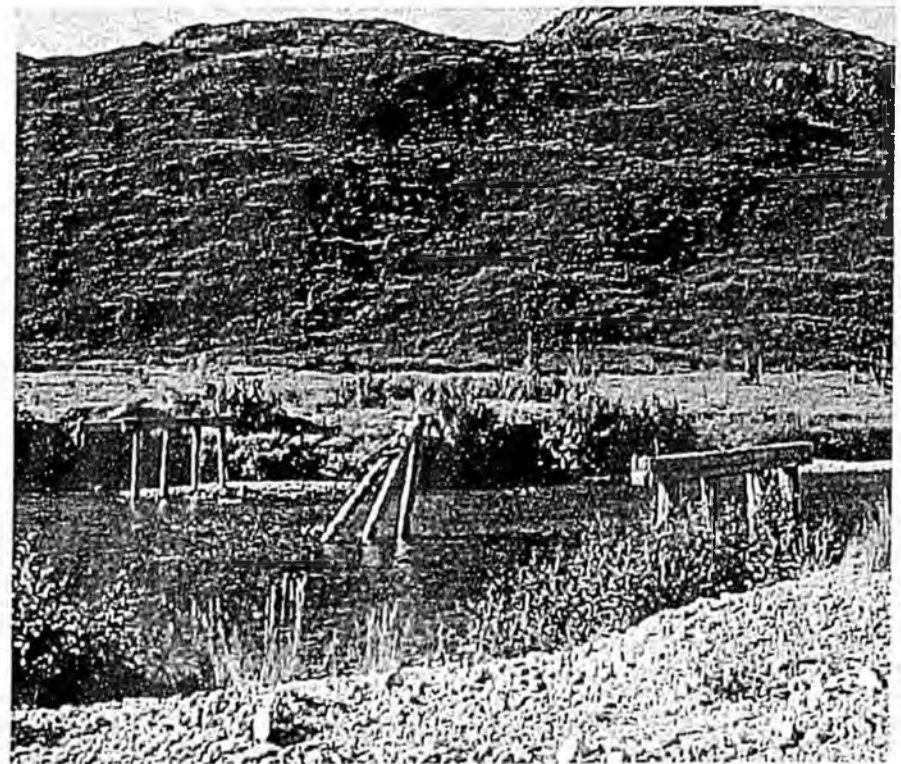
Neglected bridge, Chinkelyes Creek Williamsport-Pile Bay Road (Replaced by Bailey Bridge in 2002)
