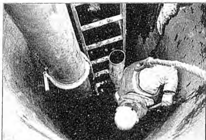
A service technician with Anchorage Water and Wastewater Utility (AWWU) works inside a caisson. Photo is courtesy of Municipality of Anchorage d/b/a AWWU.
