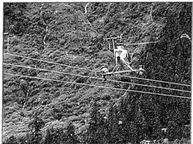
A helicopter crew replaces old aircraft marker balls on the 69kv transmission line in Juneau. Photo is courtesy of Alaska Electric Light & Power Company.
