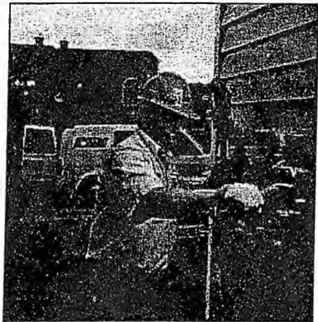
An employee for ENSTAR Natural Gas Company (ENSTAR), a Division of SEMCO, repairs a residential gas meter on a new home. Photo is courtesy of ENSTAR.
