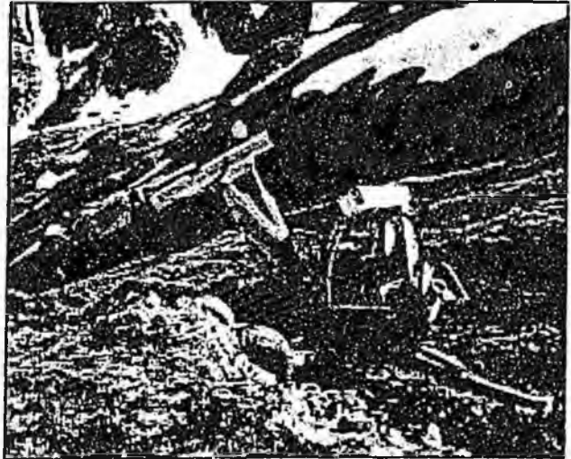
A "Menzi muck" machine carves out a trench to bury power lines. Photo is courtesy of Alaska Electric Light & Power Company.
