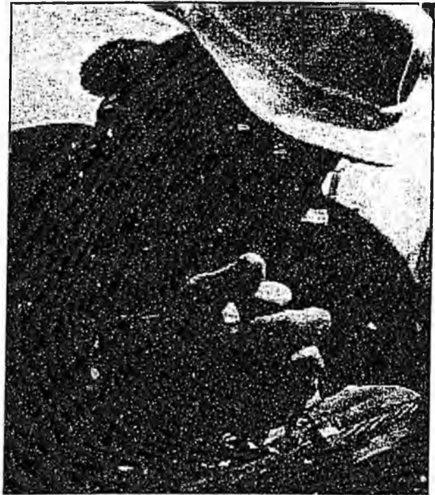
An Arctic Slope Telephone Association Cooperative, Inc. (ASTAC) telephone technician splices wires. Photo is courtesy of ASTAC.
