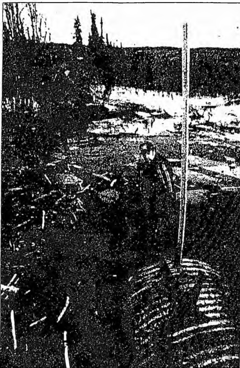
CLEARING CULVERT —Chuck Nichols, a worker for the Alaska Department of Transportation, prepares to insert a grapple hook into a culvert at 3 Mile Chena Hot Springs Road on Tuesday to clear out the dam built by beavers.
