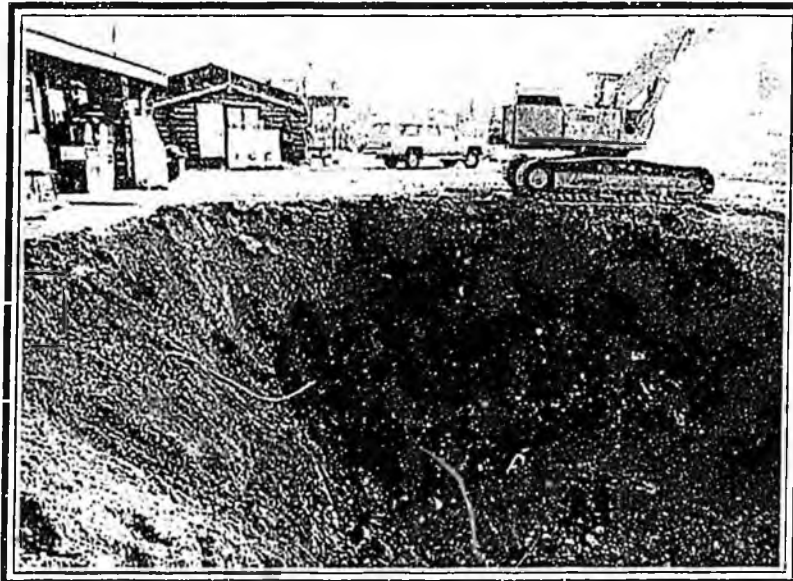
Cleanups from leaking tanks can be traumatic on Alaska's small businesses, such as this "mom and pop" facility on the Kenai Peninsula.
