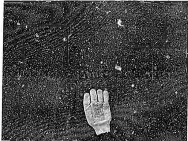
Photo No. 10 – View showing cracked and weathered condition typical of roof membrane. Complete membrane replacement appears to be necessary soon.
