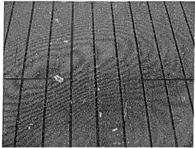
Photo No. 12 – View showing weathered siding with grooves at 4 inch spacing, and nailing occurring only at stud spacing of 16 inches along the sheet edges.
