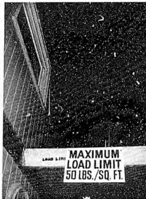
Photo No. 6 – View showing framing on the underside of the shed roof addition, and load posting of the mezzanine. The mezzanine did not appear to be used, and no fixed access is existing.
