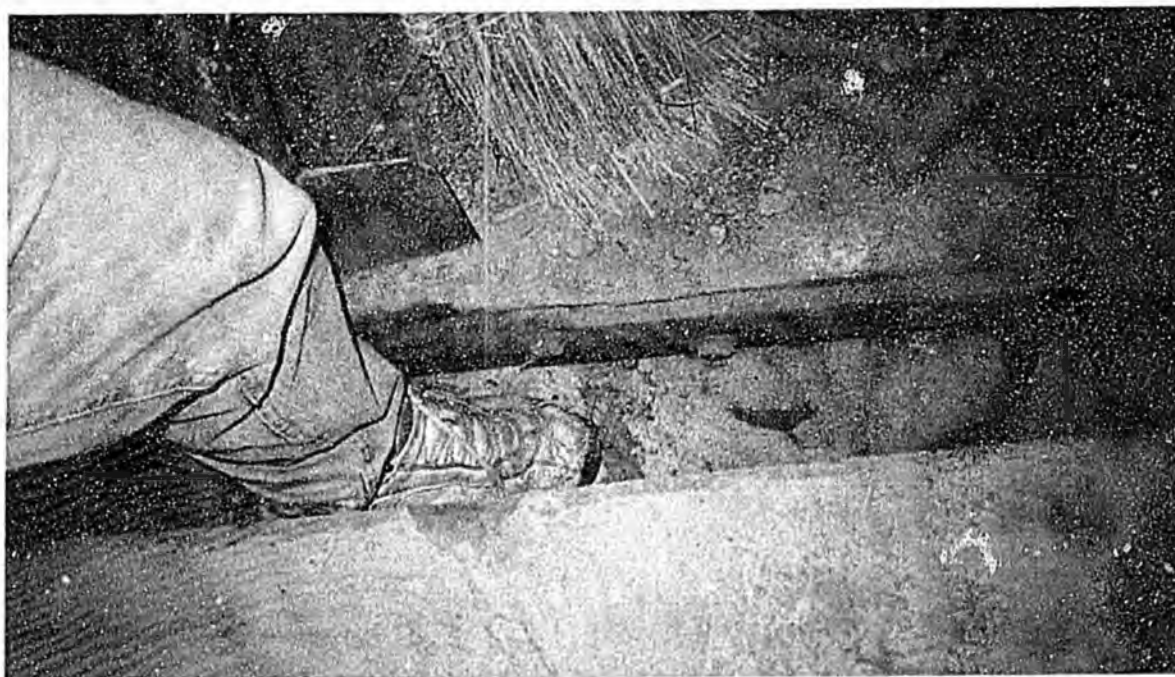
Photograph Eight: Floor slab separation and settlement.
