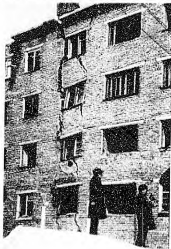
Fig. 15. Typical examples of the effects of permafrost thawing on buildings and pipelines in Siberia. Photos by S. Yu. Parmuzin.
