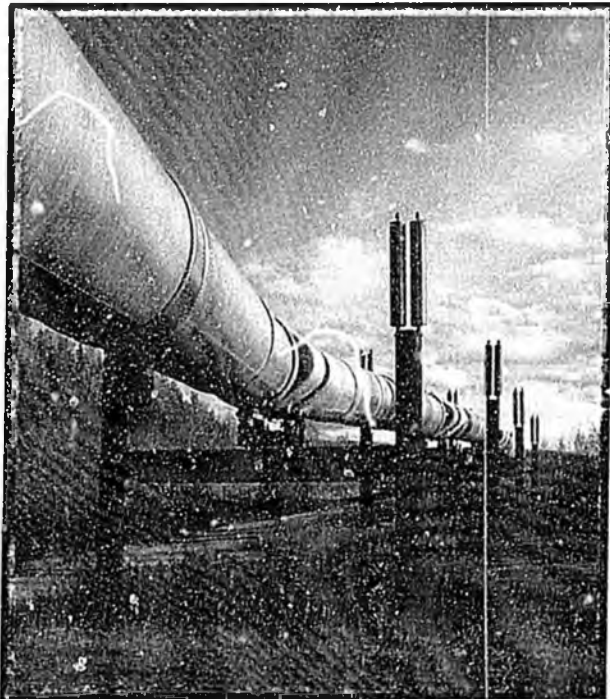
An exposed section of the trans-Alaskan pipeline on thaw-unstable permafrost ground near Fairbanks. The pipe is insulated and jacketed and rests on supports equipped with cooling fins.
