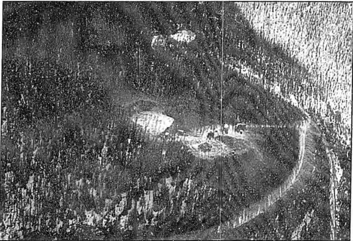
Aerial view of portal pad construction, Pogo claim area, northeast of Fairbanks. Photo Credit: Karl Hanneman
