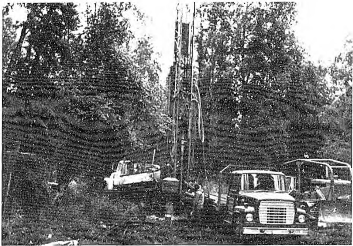
Figure 9. Drilling for coal at the Wishbone Hill project of Union Pacific Resources. (Photo by R.D. Merritt, 1983.)
