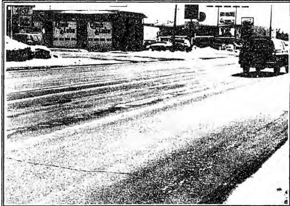
Studs have worn through the top pavement layer ( 2''\pm ) along lines spaced equally with car wheels.
