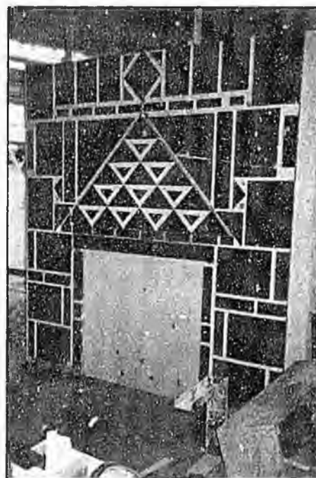
Figure 43. Jade-faced wall being built for a client by Jade Mountain Products, a subsidiary of NANA Regional Corporation. Jade Mountain designs walls and murals from jade slabs. (Photo by NANA Regional Corporation)
