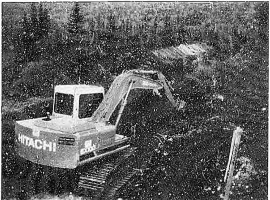
Figure 9. This excavator has been used to trace mineralization for an additional 366 m (1,200 ft) along strike at the covered Illinois Creek deposit, Kaiyuh Hills, western Alaska (Photo by North Pacific Mining Company)
