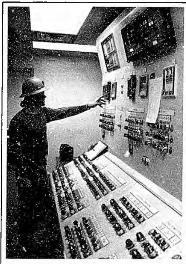
Mill Control Room at Greens Creek Mine
