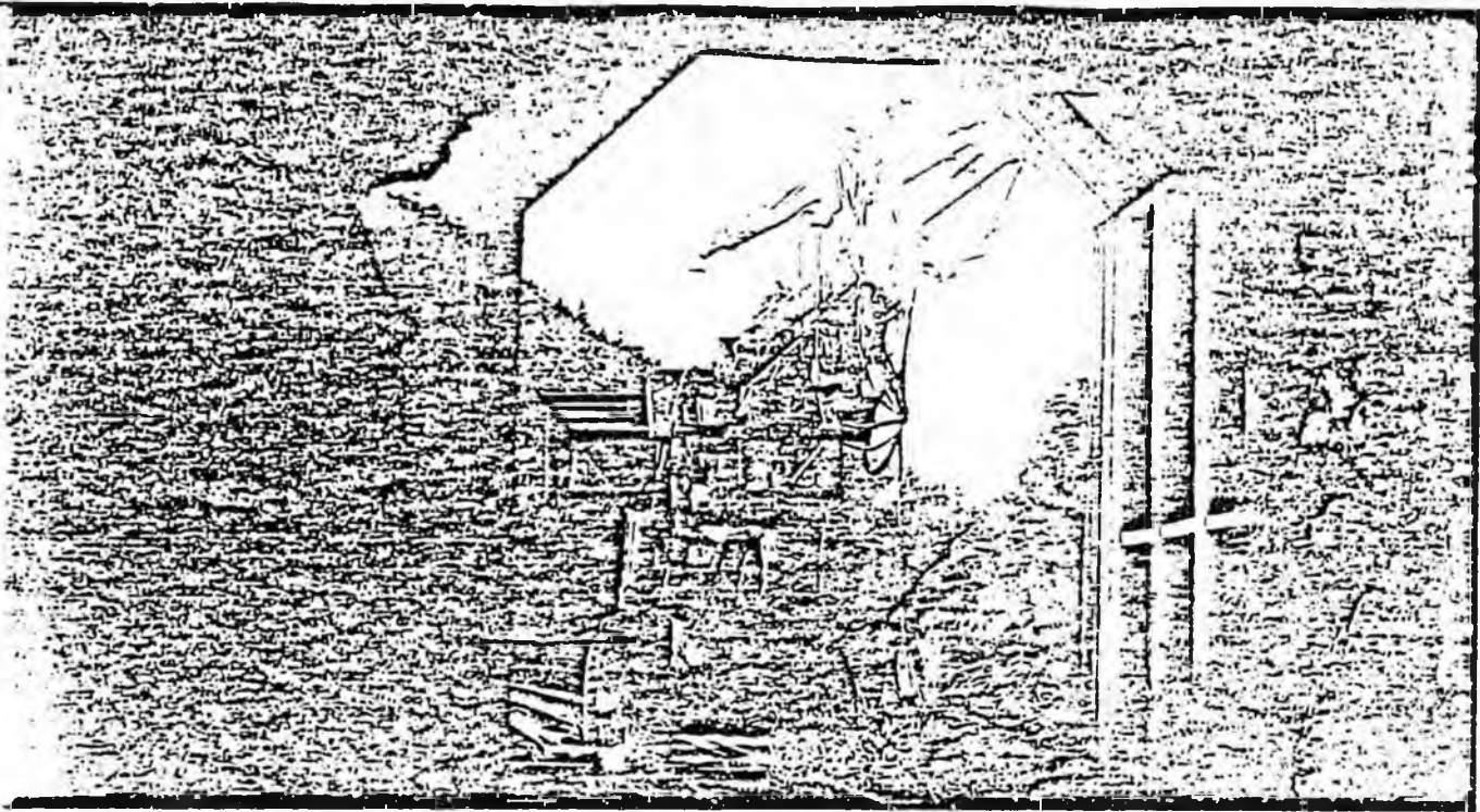
Rehabilitation of five tunnels between Seward and Portage was the single largest track maintenance expenditure in 1985. The $4 million, two-year project will be completed in 1986.
