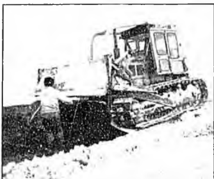
More than 1.1 million cu. yd. of geotextile was placed under the mine road, material site access roads and at bridge abutments. It was rolled out directly onto the tundra by ATVs in summer and with dozers after freeze-up. PN&D photo.
