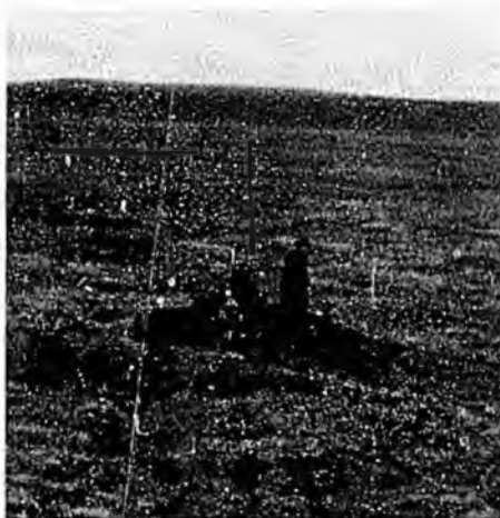
Workers lay geotextile fabric out on the tundra as work begins on the Red Dog haul road.
