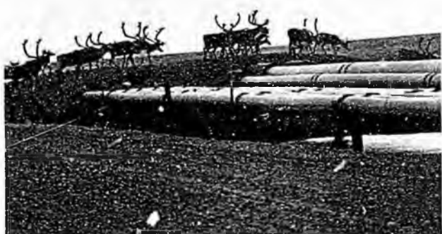
Although caribou use gravel ramps over pipelines at Prudhoe, studies have shown the ramps are not necessary.
