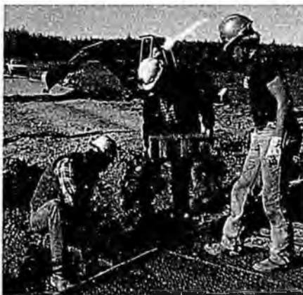
Maintenance workers installed a new, high technology material at railroad crossings that will provide a better crossing surface for the travelling public.
