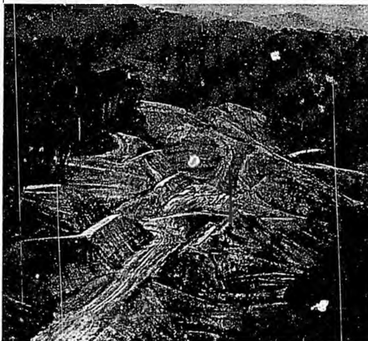
A railroad through a tropical rain forest—the Transgabon railway under construction between Owendo and Franceville.
