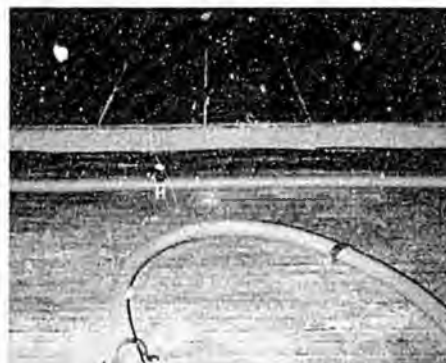
Close up shows a portion of the first floor before the concrete was poured and another area where glazed Italian tile covers the slab.
