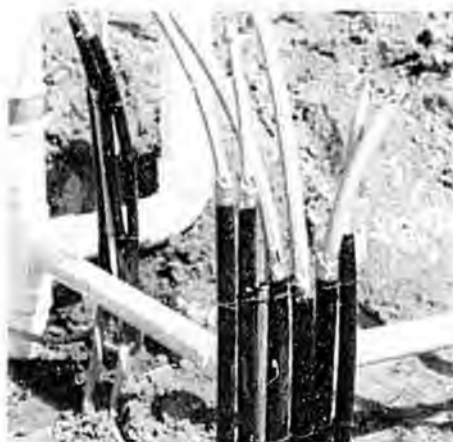
Protective polyethylene sleeves are slipped over the polybutylene pipe and they are secured to a metal stake to prevent movement during the pouring of the slab or damage to the pipe during final stages of slab construction.
