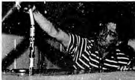
Tom Puckett pulls back the insulation to reveal one of the 3/4" gray Duraflex polybutylene lines linking solar collectors with a 500-gallon Aqua Stove water tank.
