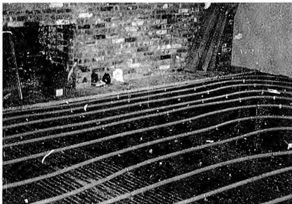
Three-hundred-foot coils of 1-inch pipe were embedded in the first floor slab. Pomanowski said the system also served to effectively radiate heat into the basement.
