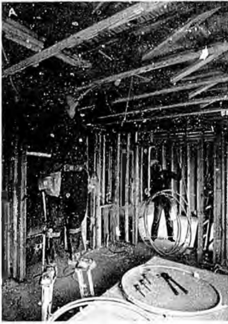
Two installers unroll a coil of polybutylene pipe along ceiling beams in an apartment at Alpha Point. A smaller coil, crimping tool and pre-fabricated drop pipes to sprinkler heads are visible in the foreground.
