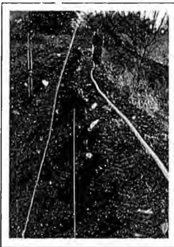
A long run of 2-inch Duraflex polybutylene square pipe lays flat alongside a trench with virtually no tendency to recoil.
