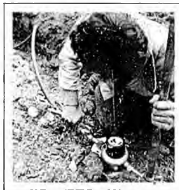
A fitting is tightened just prior to a pressure test at 40 gpm. Water service lines of Duraflex polybutylene pipe are blue coded for easy visual identification in common trenches.
