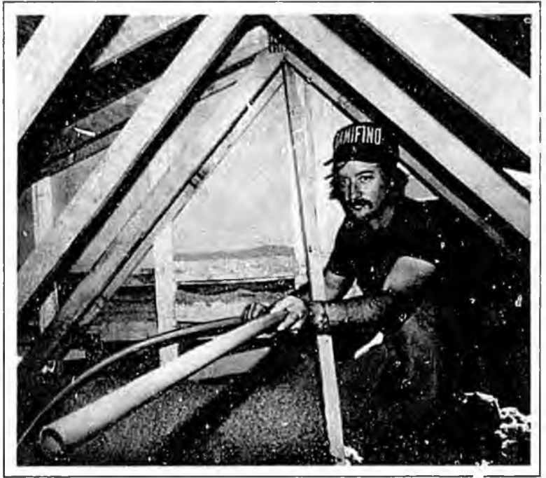
Sections of lightweight polybutylene pipe were connected outside, then easily fed through an attic opening, greatly reducing the time required to install a sprinkler system for the Scottsdale tests.
