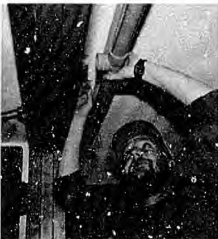
A heat fusion tool is used to connect the feeder pipe in the hall to the line extending to the sprinklers in each room.
