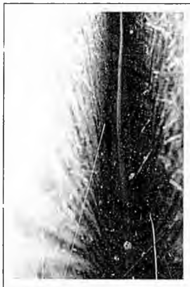
The key component of a closed-loop, earth-coupled heat pump system is polybutylene pipe shown here just before being covered in the bottom of a 6-foot trench.
