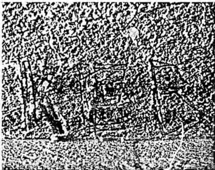
Friable Material That Has Been Scraped
