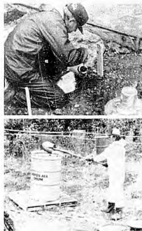
Soil contaminated with PCB's was removed this past summer from an area near the new Aniak school. Workers dug up enough tainted dirt to fill two C-130 cargo planes. The area is now secure for the winter. The discovery of the inadequate cleanup of this abandoned air force site has led DEC to reinspect other sites for possible contamination. Here DEC's Jim Allen (top photo) and helpers take samples and collect soil for shipment.
