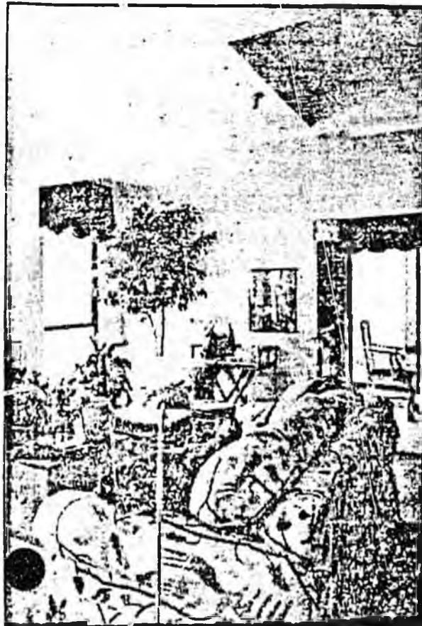
WATERFORD PLACE: Sprinkler in Cobb home.
