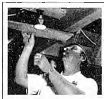
Fire Inspector Ed Harrod checks installation of fire sprinkler specifically designed for residential use.
