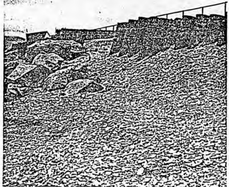
This seawall was constructed behind the school sewage lagoon in an attempt to slow erosion during storms.
