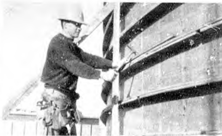
Securing this large circular form in preparation for a concrete pour is part of a day's work for this apprentice.
