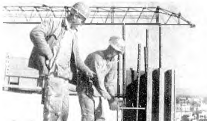
A carpenter apprentice, working with a journeyman carpenter on a reinforced concrete form job.
