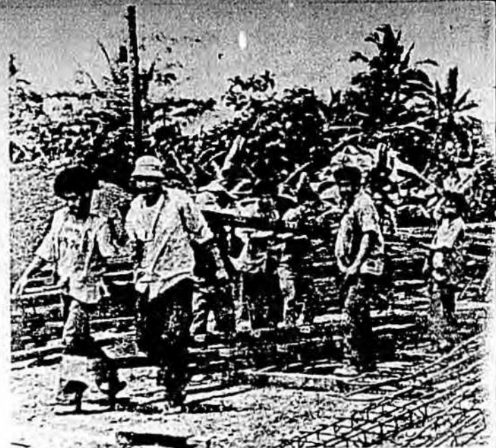
Construction work in progress on the Telecommunications Project in Apia, Western Samoa.
