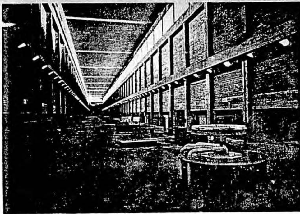
FOURTEEN 100,000-KILOWATT GENERATORS housed in this plant at Juplá Falls on the Paraná River help power farm, industry and home in the Greater São Paulo area of Brazil. Juplá and the Ilha Solteira plant will form 4.6-million-kilowatt complex. Both have received Bank financing.
