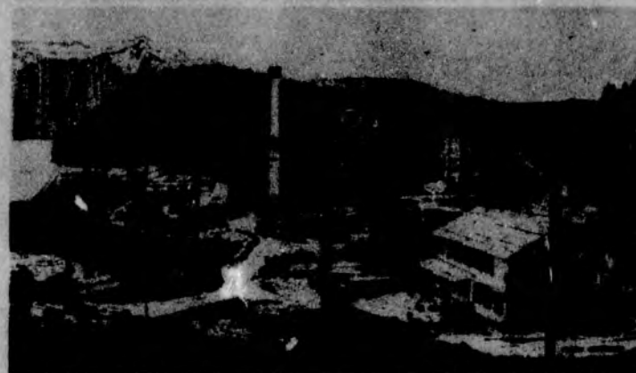
Powerhouse stack, machine shop, dock, pulp preparation building, pulp storage building and sulfur silos taking shape - May 21, 1953.
