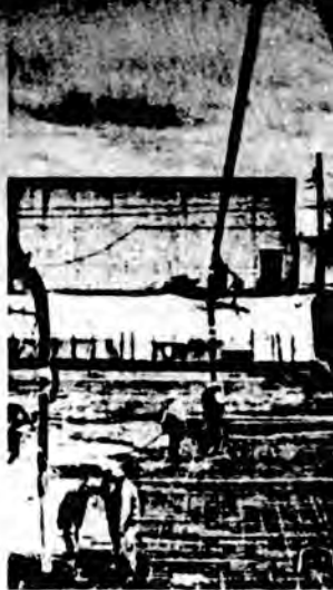
Ken Brady Construction Company's crew working on Alaska's largest single concrete pour ever made. It will be the main foundation of the new International Brotherhood of Electrical Workers Trust Tower.
