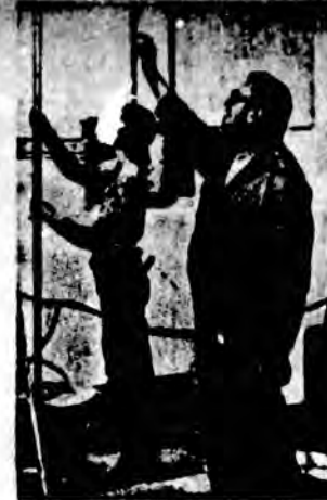
Mike Steffens instructs Lois Haper in the procedures of insulating the new Anchorage Federal Building. Both are in Asbestos Workers Local 97.
