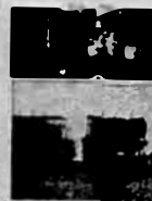
High pressure sour gas re-injection train, Hesse Processed Plant, 477 bar
