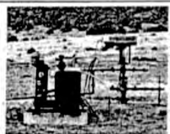
Water Pump and gas Engine
