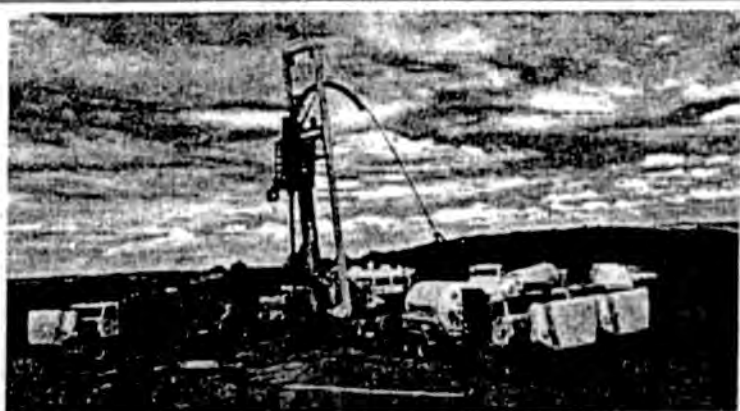
Evergreen Frac Equipment - uses mostly nitrogen gas
