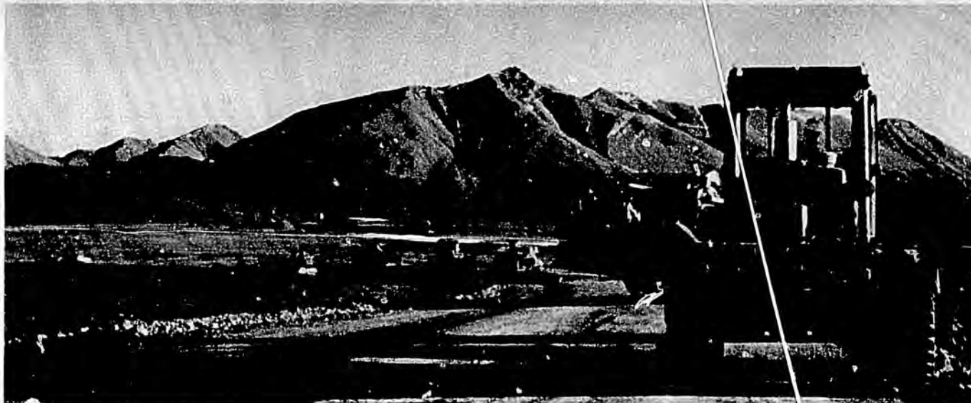
COMPLETION of the base for the 360-mile Alyeska haul road to the North Slope paves the way for intensive construction work on the line next year—and for a major boost in domestic oil supply in 1977.
