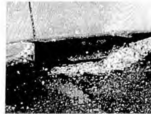
Fairbanks Health Center, Sidewalk Erosion
