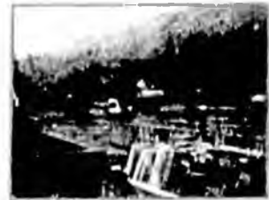
Construction site for the new Denali Commission building, which will house the Bring the Kids Home Focus Area.
