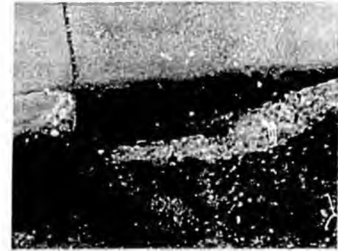
Fairbanks Health Center, Sidewalk Erosion
