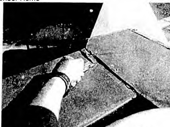
14. Failed sealant at poor quality flashing detail on parapet caps
