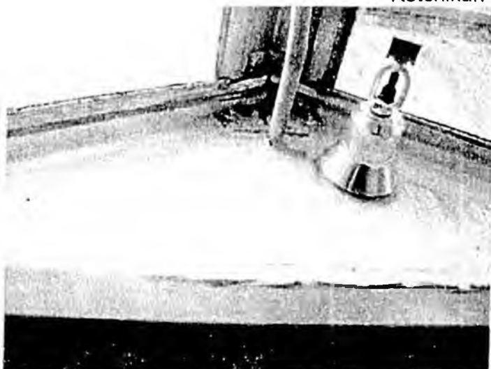
13. View of sealant applied to inside the greenhouse to walls & door frame. Note water stains.
