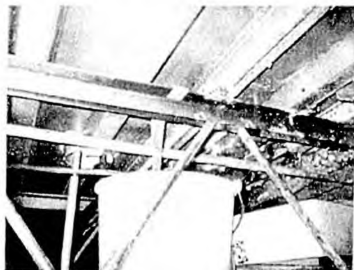
12. Leak #1, Deteriorated steel deck under greenhouse and mechanical room
