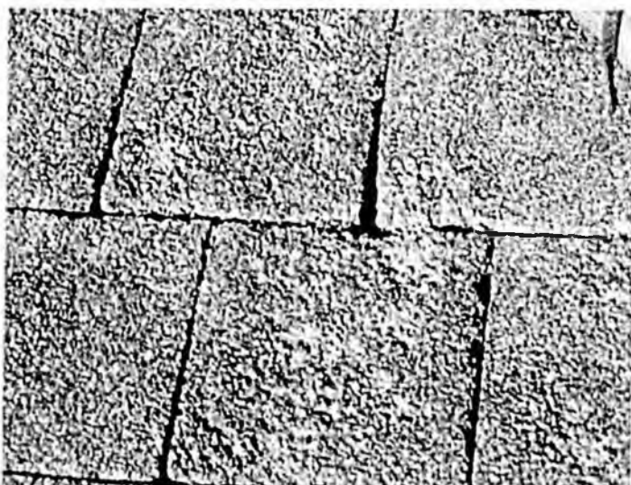
15. Erosion of the ballast pavers
