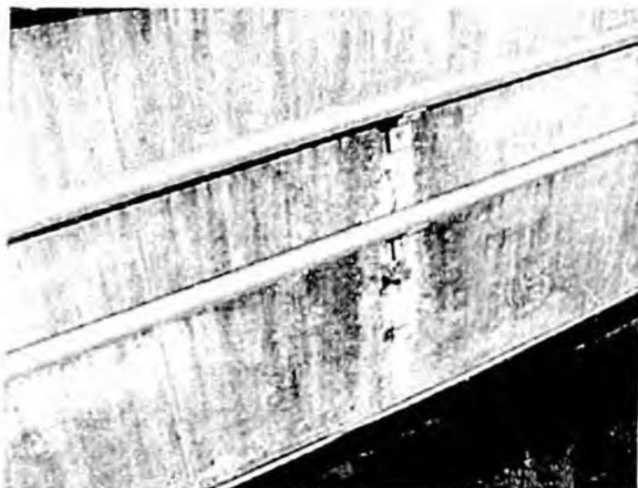
9. Erosion of unpainted cement board siding along ramp
