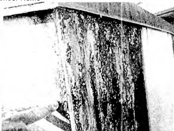
8. Erosion of unpainted cement board siding
