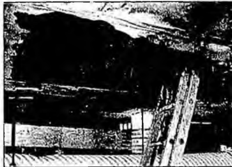
Schools In Peril Hooper Bay High School, Lower Yukon, shows rotted structural members. Extensive deterioration was discovered in the area of the bathrooms and showers during an appraisal in February 2001 by SERRC, Inc.
