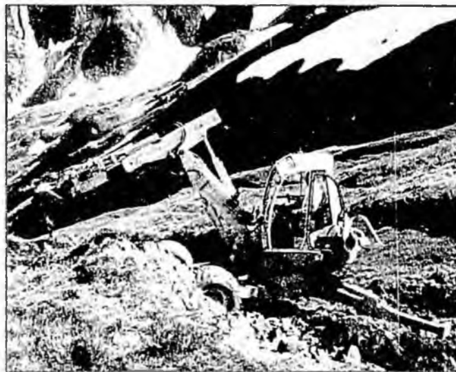
A "Menzi muck" machine carries out a trench to bury power lines. Photo is courtesy of Alaska Electric Light & Power Company.
