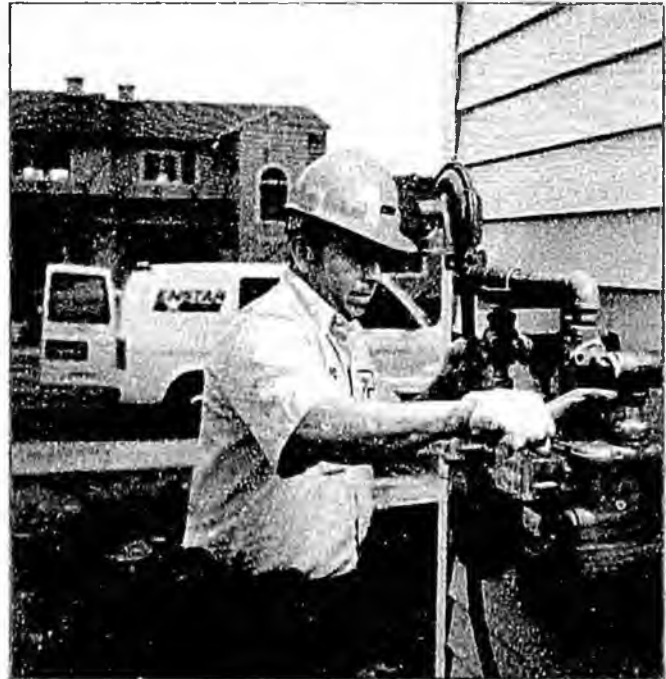
An employee for ENSTAR Natural Gas Company (ENSTAR), a Division of SEMCO, repairs a residential gas meter on a new home. Photo is courtesy of ENSTAR.
