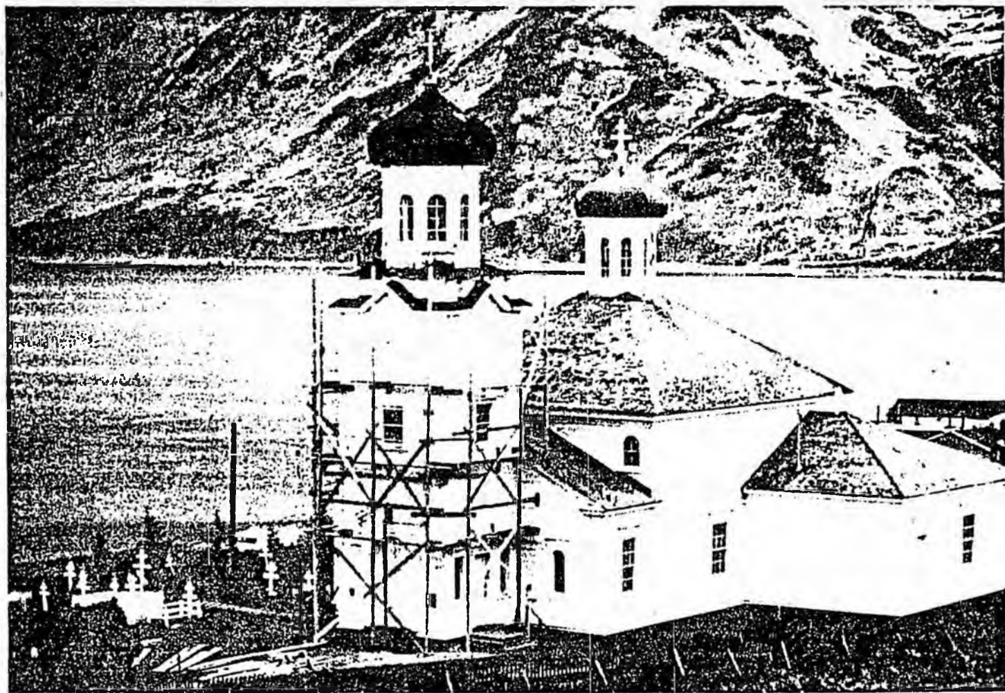
Although maintenance work is done on a continuing basis, severe weathering conditions and structural problems threaten the long-term preservation of this magnificent church. Photo: CCC Architects
