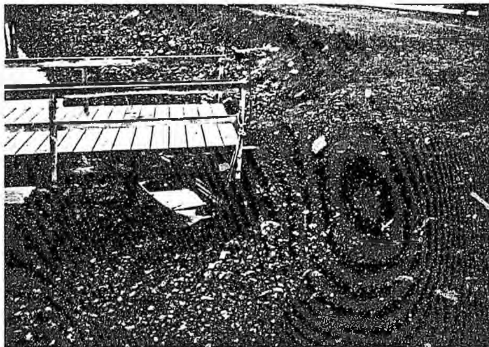
Figure 3. Photograph of the eroded shoreline in the Seldovia Small Boat Harbor.
