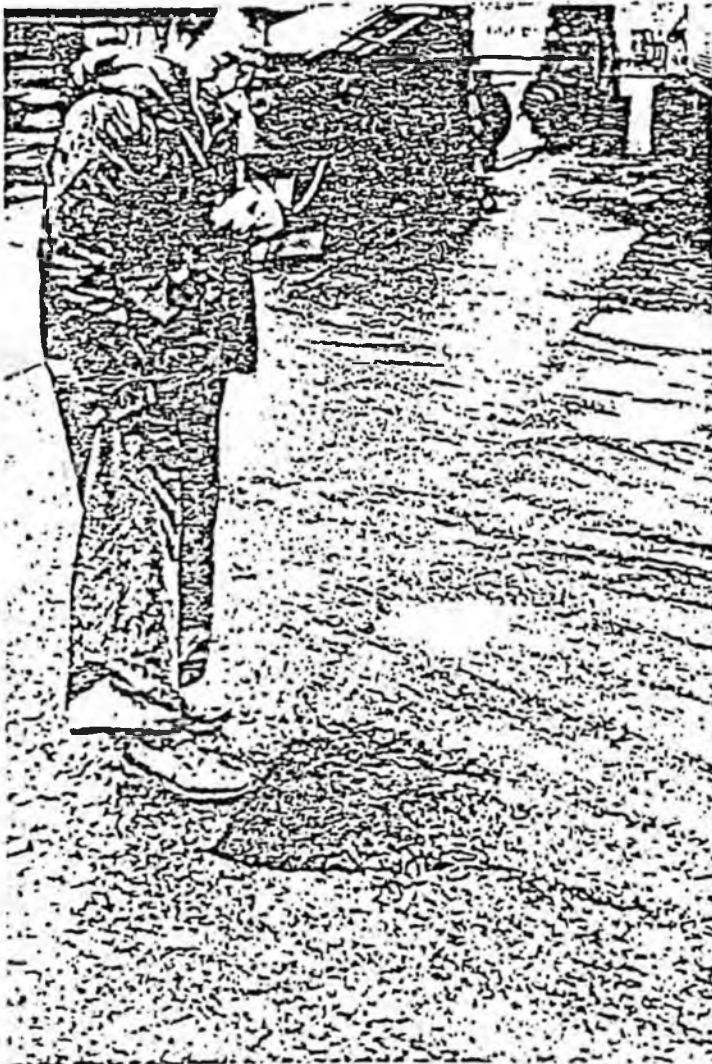
Photo No. 21: Sinkhole in rockfill in back of wharf. Typical three places along easterly third of wharf.
