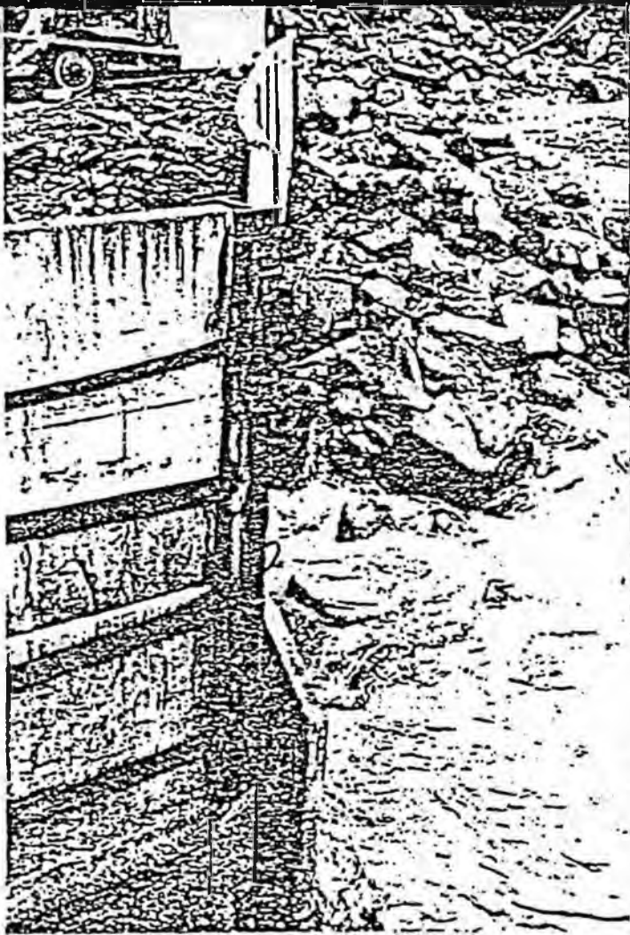
Photo No. 14: View looking northeasterly along top of east wingwall. Note irregular alignment of wall top.
