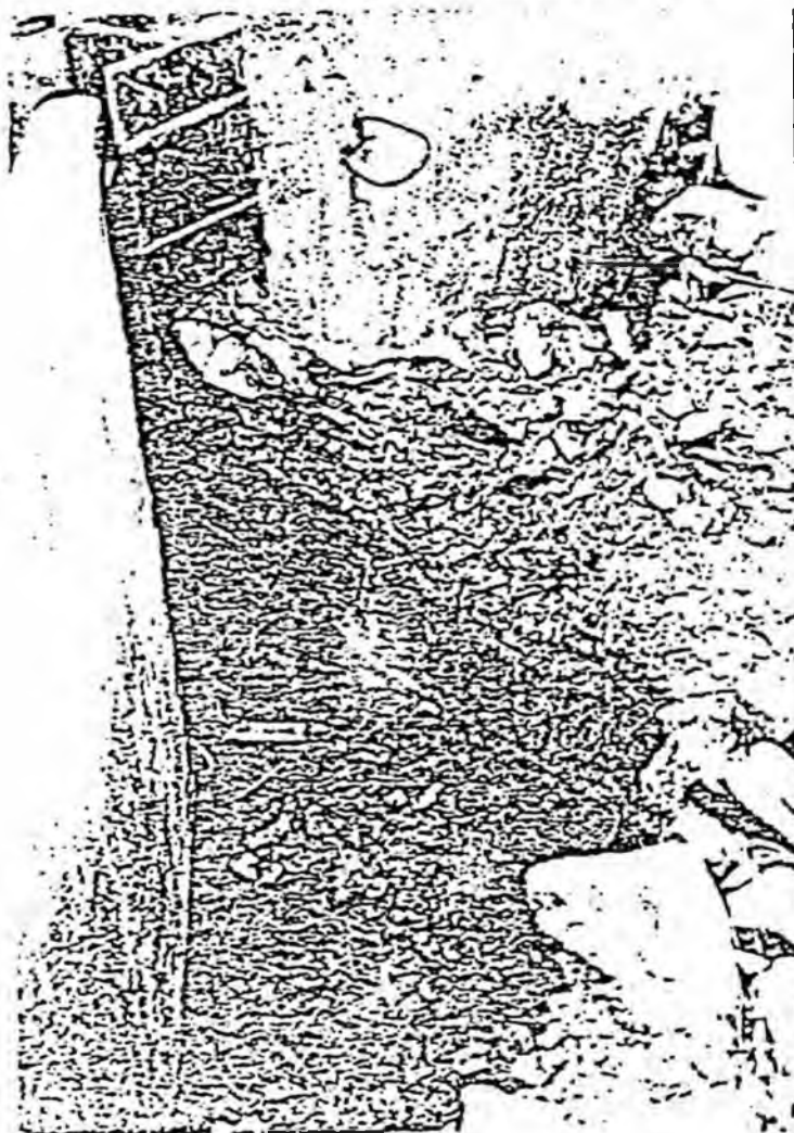
Photo No. 15: View at corner pile, inside of east wingwall. Due to broken tierods, pile is retained in place by buried steel tension beam installed by City of Kodiak. Loss of fill material caused by wave action through loose panel below.
