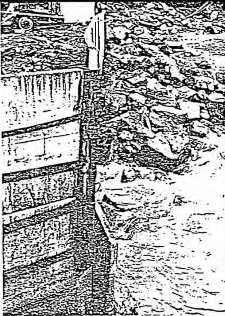
Photo No. 14: View looking northeasterly along top of east wingwall. Note irregular alignment of wall top.
