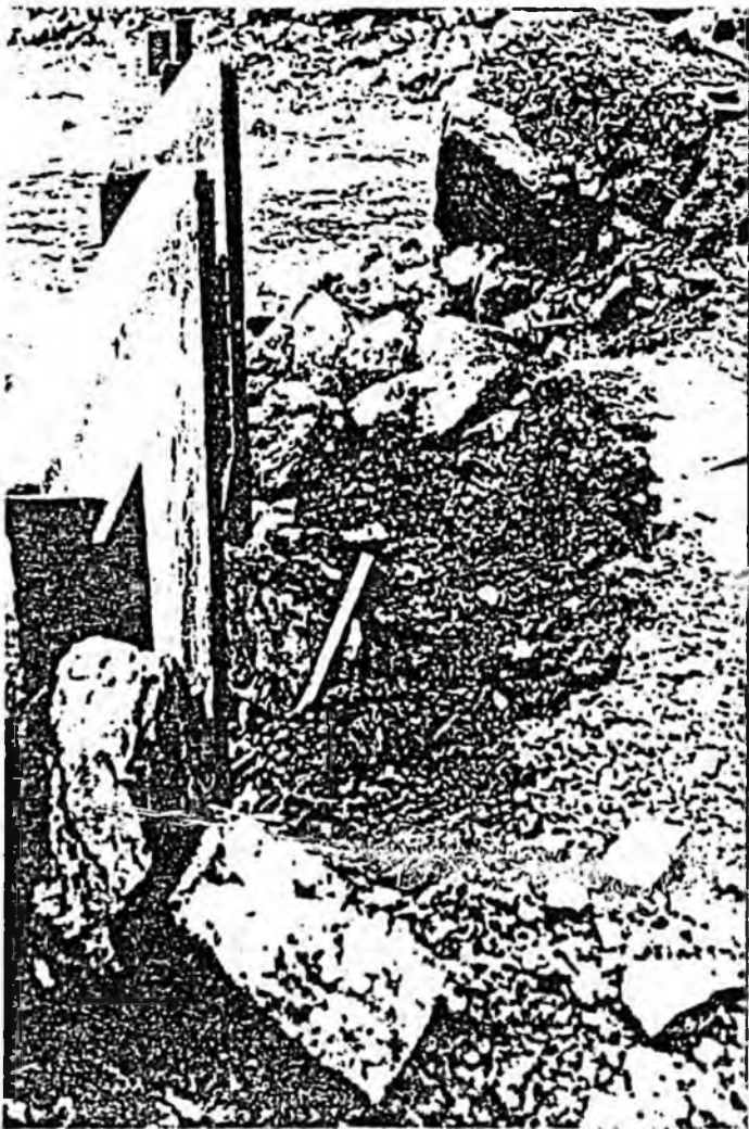
Photo No. 19: View of northern end of west wingwall looking north. Fill washed out from behind wall by storm waves.
