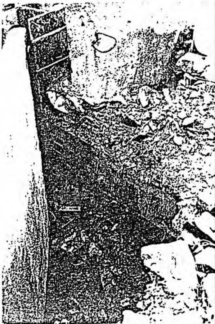
Photo No. 15: View at corner pile, inside of east wingwall. Due to broken tierods, pile is retained in place by buried steel tension beam installed by City of Kodiak. Loss of fill material caused by wave action through loose panel below.
